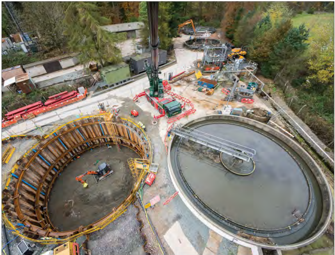
Photograph Above. A good construction site. It doesn't get much more picturesque than this.
