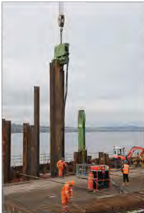
Photograph Above. A Piletec attachment used for driving sheet piles in Dundee
